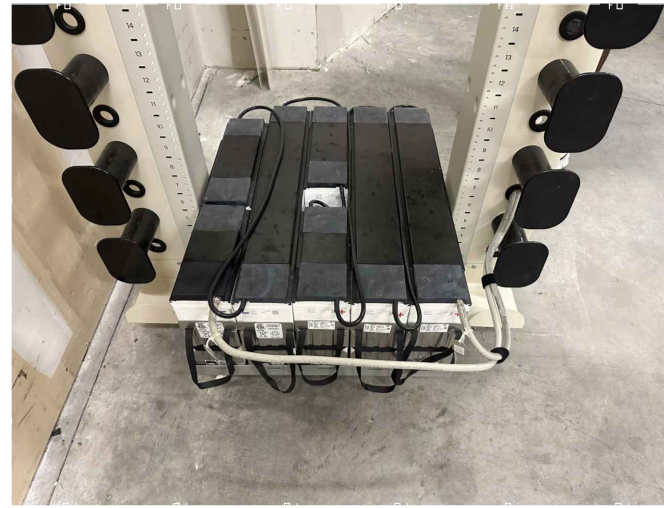
7 PHOTO - VZW RACK VIEW: LOOKING NORTHWEST
