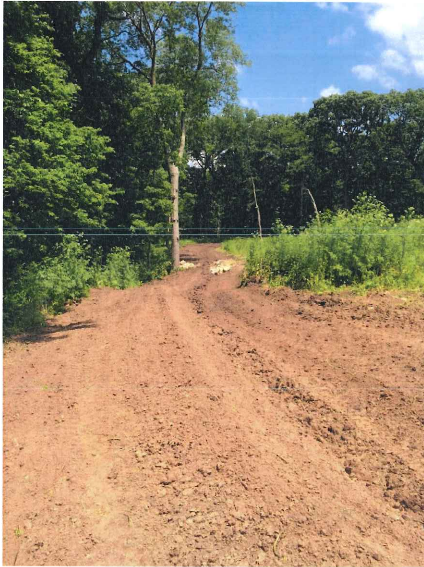
Existing Linear Silt Trap
